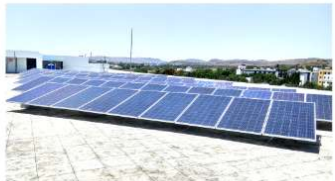
Solar roof top Photo - Voltaic Project
